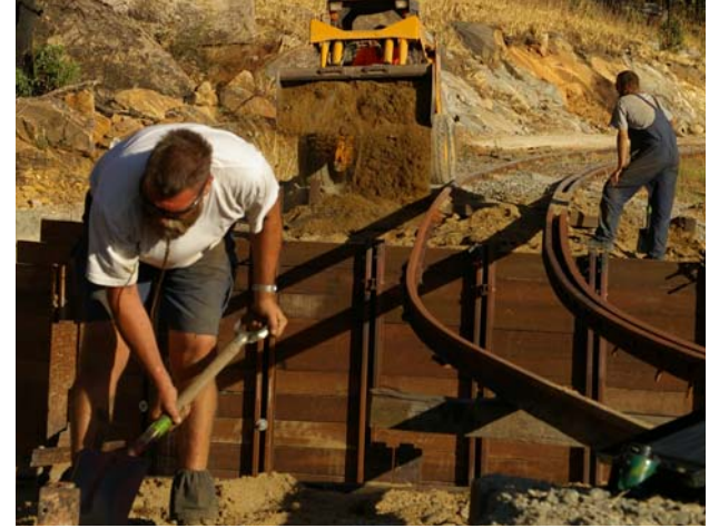
Work on 13km bridge continued thanks to the purchase of a Mustang bobcat.
