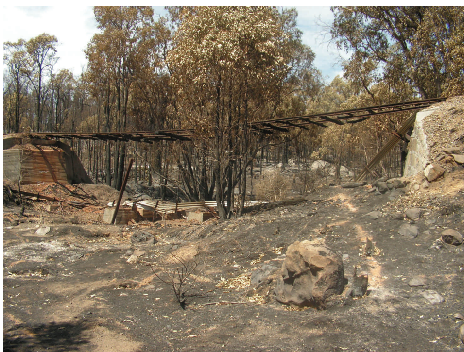
16km bridge – After being ravaged by bushfire
